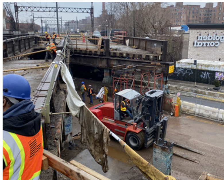
Crews work on the demolition of half of the existing bridge at Bronxdale Avenue Bridge. February 2024.
