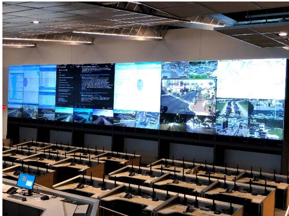
New Video Wall in Bus Command Center (East Side)
